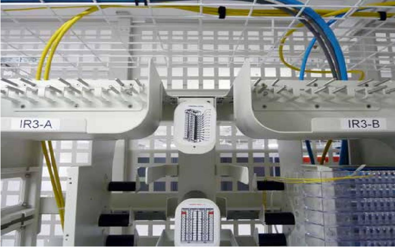
Corning EMF Rack.
