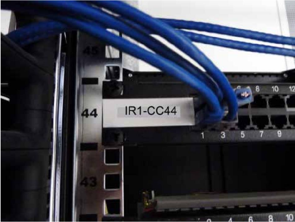
Tyco NetPodium Rack – Patch Panel.
