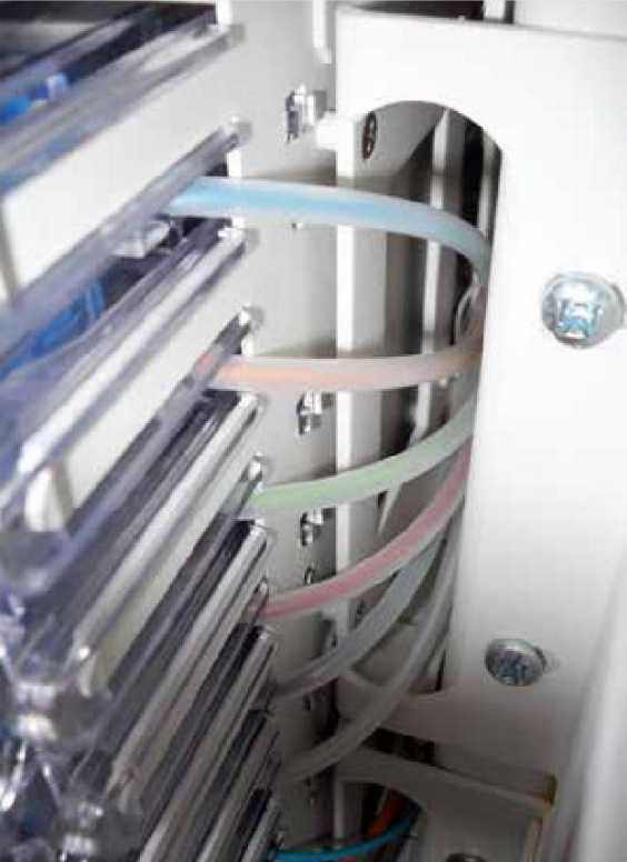
Loose tube fibres protected by transport tube.
