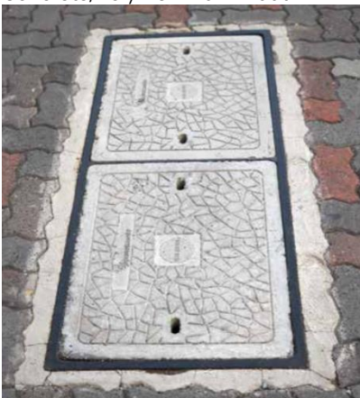
Concrete/Polymer Draw Pit at B1.
